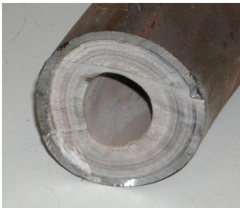
Scale formation in pipework
