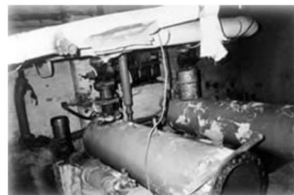
Damaged asbestos lagging
