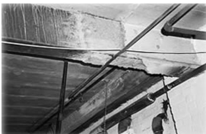
Sprayed "limpet" asbestos
