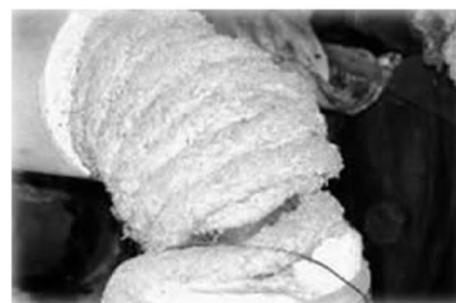
Asbestos rope and lagging
